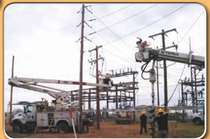
Crews energized a new substation in Tunnel City, improving reliability and splitting loads.
