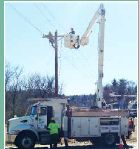
A seven mile three-phase line between the Clifton and Plymouth substations was rebuilt.
