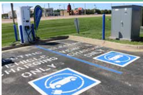
The first public electric vehicle charging station in western Wisconsin.
