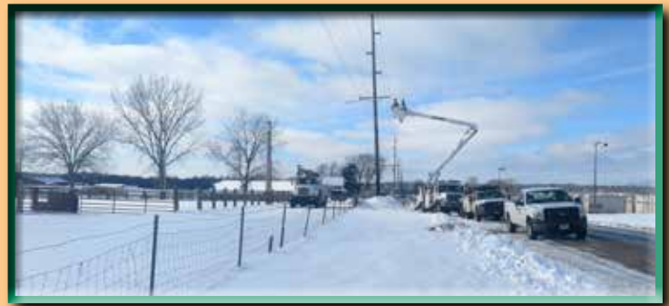
A one-mile line rebuild was completed on Grain Avenue, Tomah, to provide service to Mill Haven Foods.
