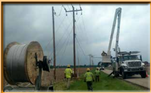
Construction crews rebuilt the lines that feed into the Tunnel City Circuit 3.
