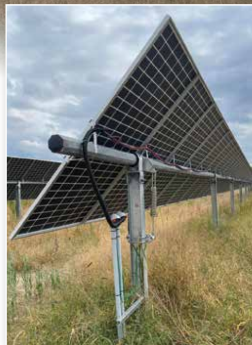
Bifacial solar panels allow energy to be absorbed from the sun reflected off the snow in winter months.
