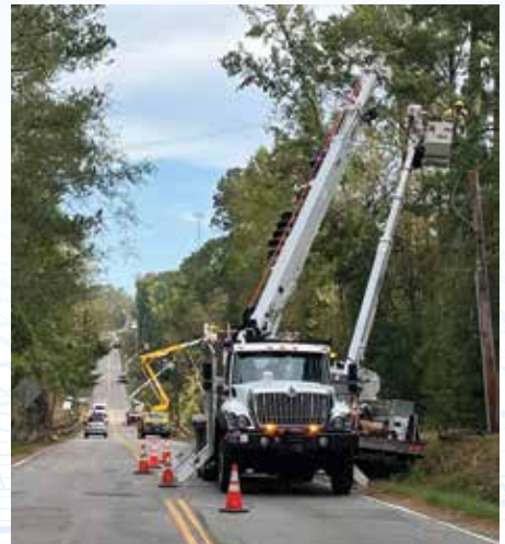
A line of Wisconsin co-op trucks and crews working on repairing a three-phase line.
